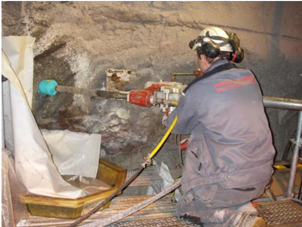
TASI-tunnel, drilling before installation of casing in one of the holes for the coming TASS-tunnel (photo Oskar Sigurdsson)
