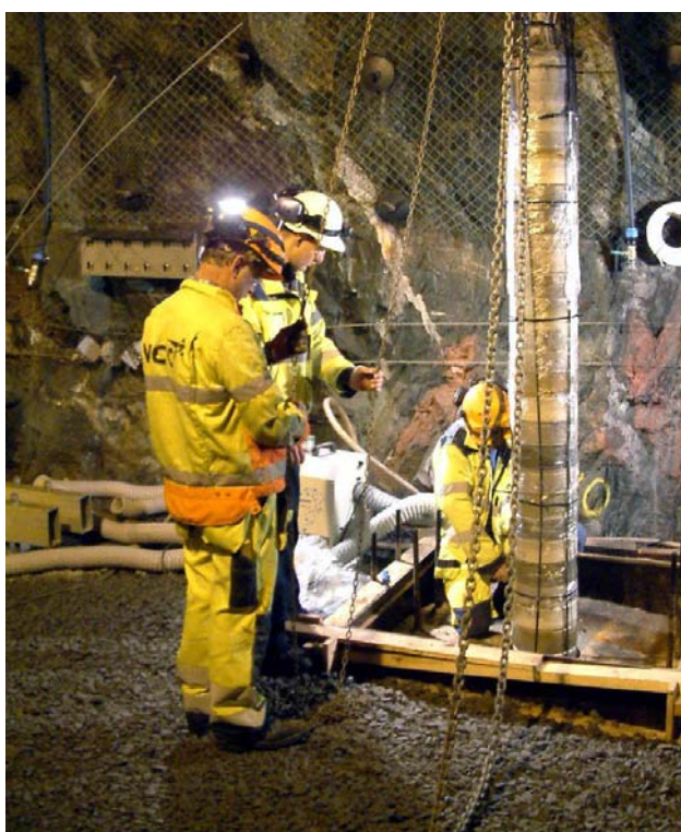
Installation of one of the three packages illustrating the mixing of the different compacted buffer discs.
